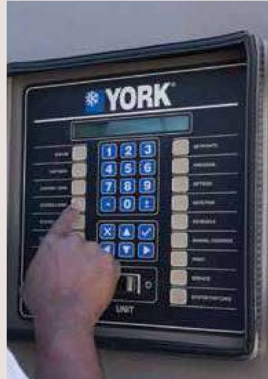
TOTAL FACILITIES MANAGEMENT
